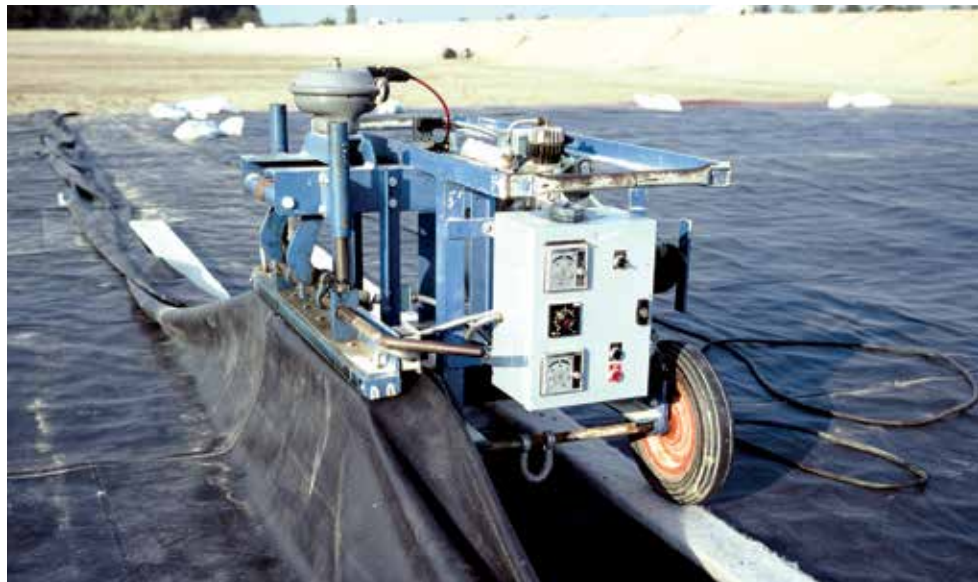
FIGURE 13 Butyl rubber geomembrane seaming machine (photo taken at a different site in the 1970s). The same machine is seen on the slope in Figure 10. The seaming configuration shown in Figure 12 was used both in the factory and in the field with the same jaw size.
