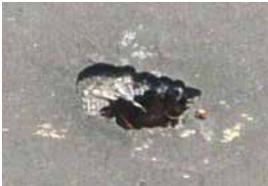
FIGURE 15 Hole in the geomembrane with reinforcing fabric (scrim) visible on the left side of the hole.
